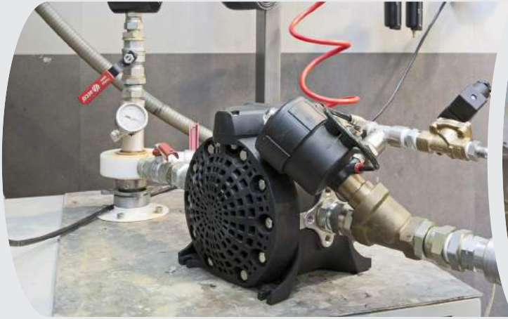
Cement additive dosing.
