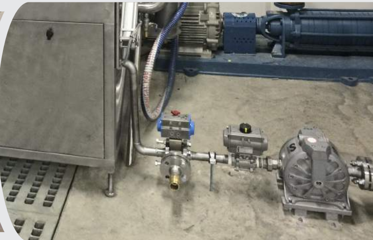
Chemical products dosing.
